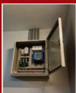
Gateway Box Underground Tank
